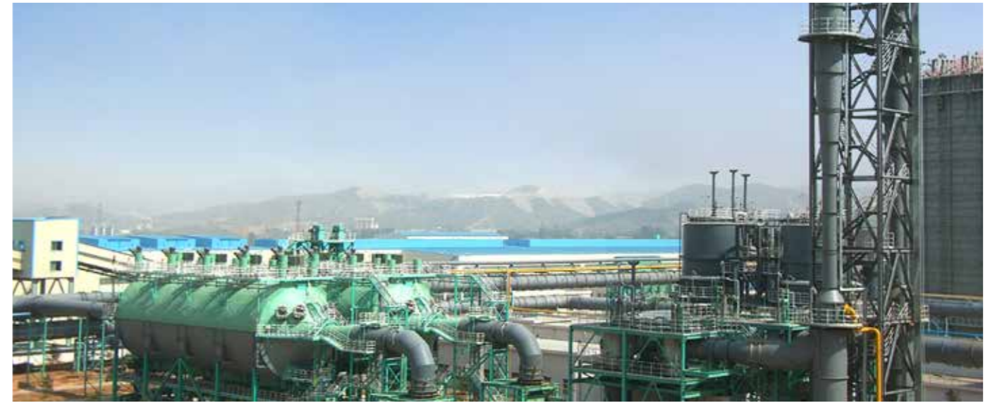
LD(BOF) gas recovery system
