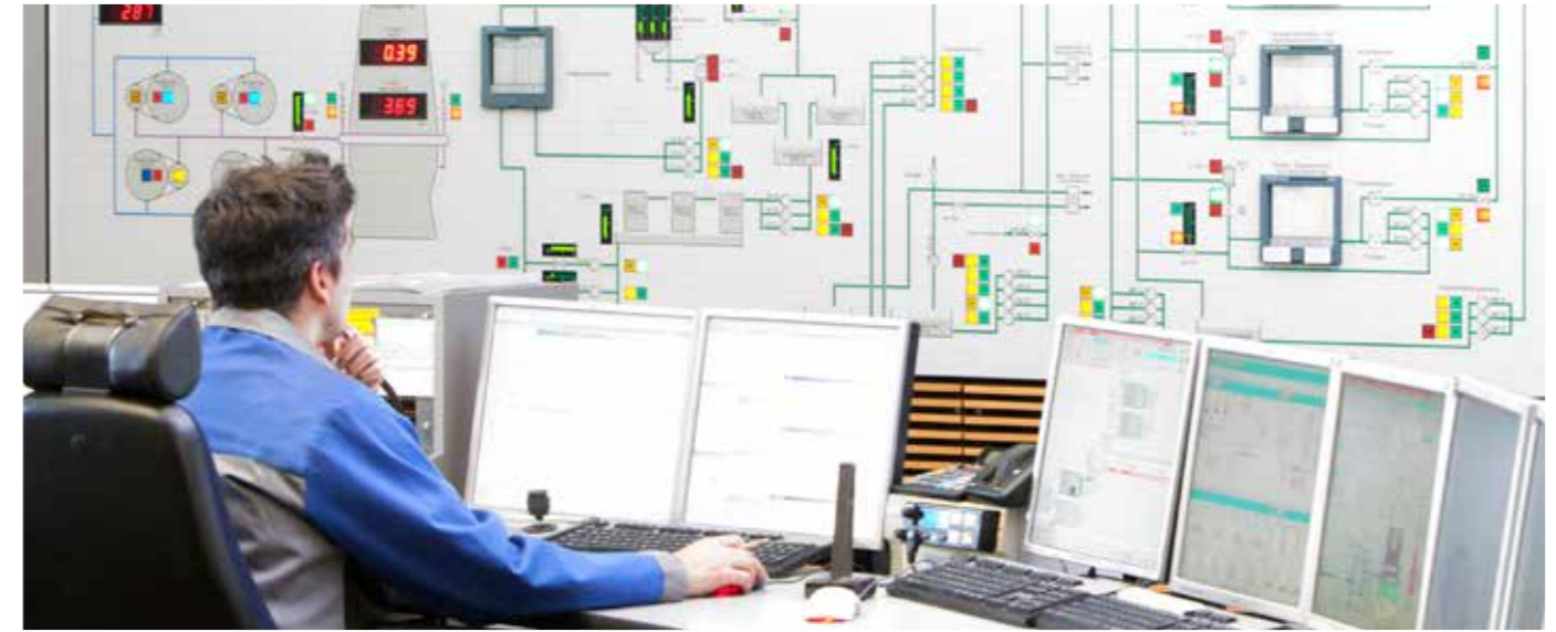
BF Optimization - blast furnace control room
