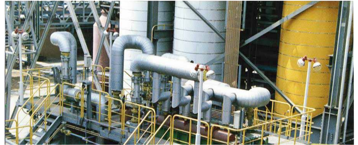
Blast furnace stove heat recovery
