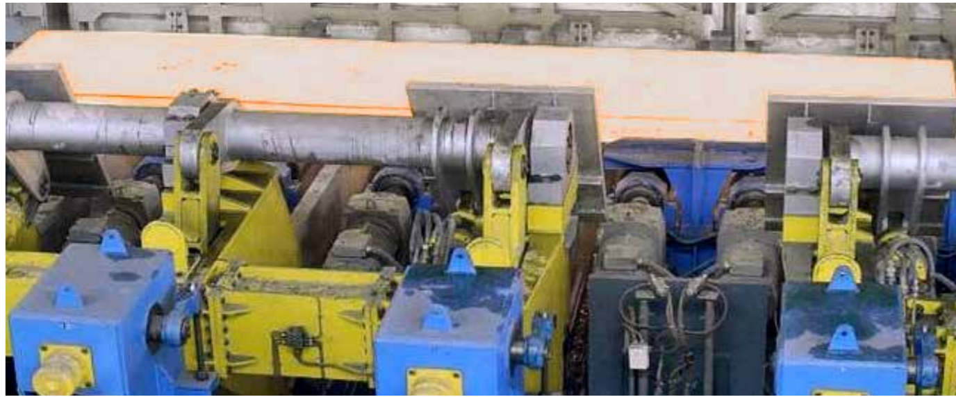
Primetals Technologies Furnace Optimization
